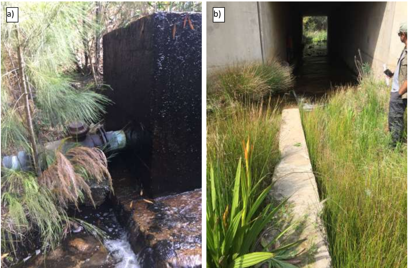
Figure 3.4 The 200mm diameter pipeline extends from a) the pool structure associated with the weir for diversion of runoff from the Huiskloof River and b) then crosses the active channel of from Huiskloof River immediately upstream of the culvert below the R43.
