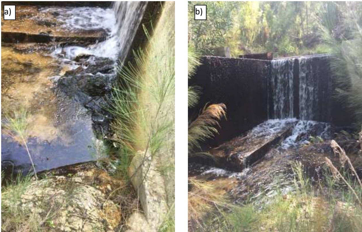
Figure 3.2 The weir constructed on the Huiskloof River in 2010 a) showing the bedrock outcrop on which the weir is situated thus minimising the risk of erosion an b) looking upstream from the active channel
