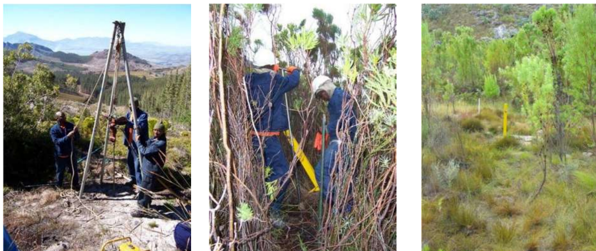
Figure 3.1. Air percussion drilling, hand augering and final installation of piezometers (note that in the photo on the left the piezometer is located within a firebreak on an existing footpath).
